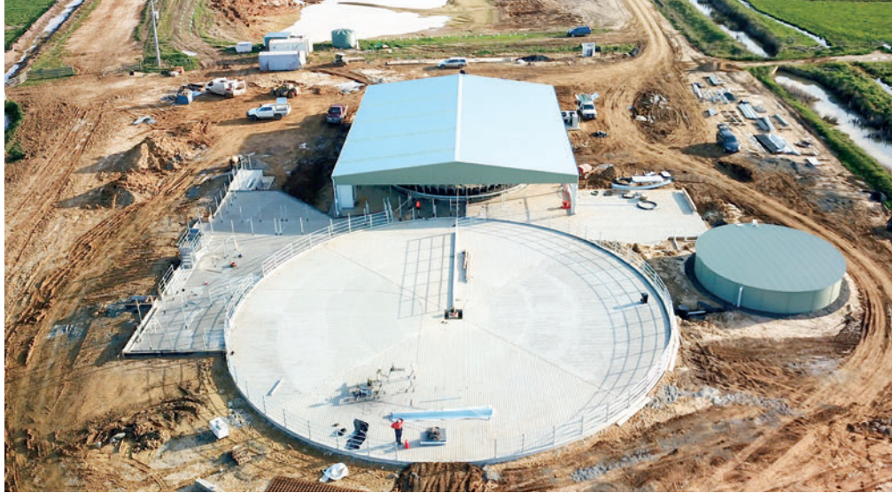
Once the decision to build is made, the next choice is whether to do it on an existing site, or to break new ground.
